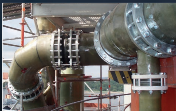
Ring piping made from PP/FRP for the flue gas scrubber in a power plant.
