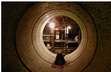
Left: Ring-lined, multilevel rotary kiln lining with 10% chromium-corundum brick.
