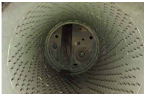
Left: Large-area use of carrier bricks in a newly lined rotary furnace (diameter: 4800 mm).
