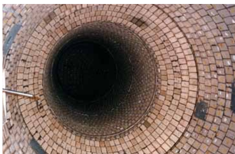
Left: View in a round post combustion chamber lined with andalusite bricks.
