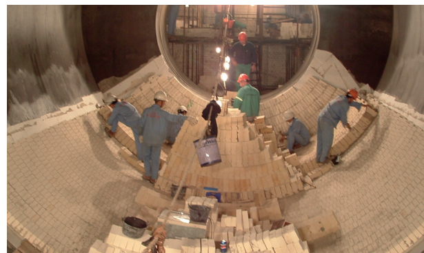
Above: Multi-layered brick lining of the horizontal chamber with the torospherical head connection to the vertical furnace of a sulphuric acid cracking plant
