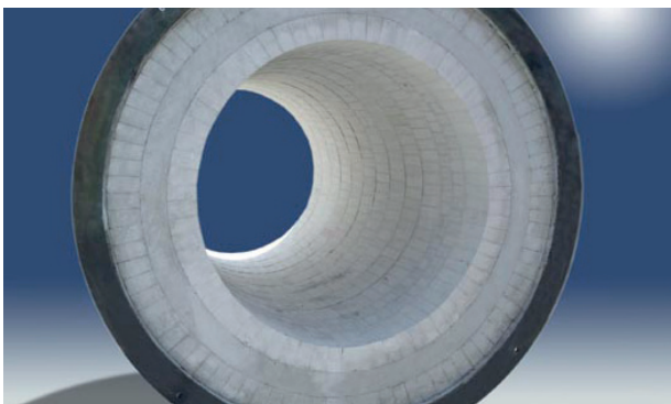
Above: Multi-layered brick lining of the horizontal chamber with the torospherical head connection to the vertical furnace of a sulphuric acid cracking plant
