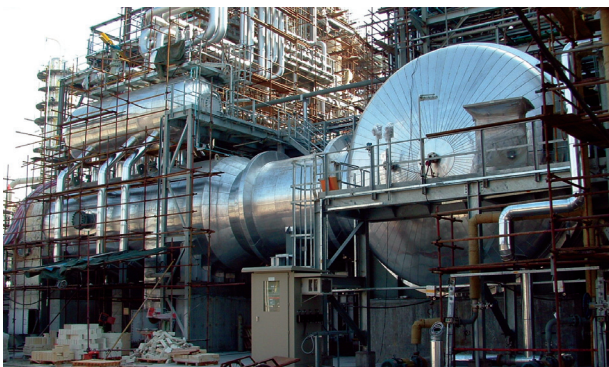
Above: Site view of the horizontal chamber and waste heat boiler with the vertical cracking chamber.
