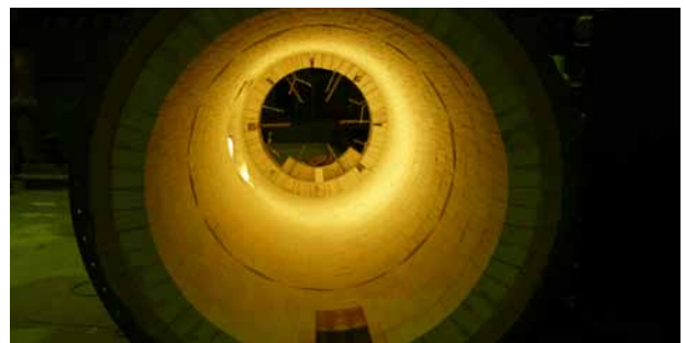
Above: Upper section of a reactor with three-layer wall construction and monolithic ceiling mounted with anchors.
