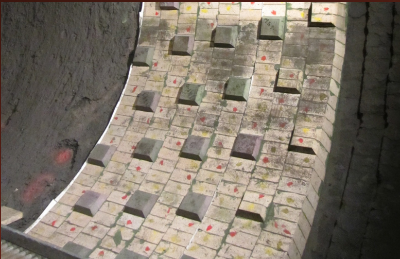
Fig. 2: Inlet zone of the rotary kiln newly lined with andalusite bricks and lifters.
