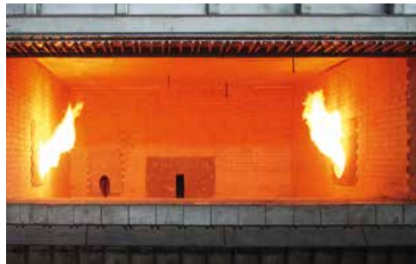
Above: Trolley melt furnace with brickwork wear lining
