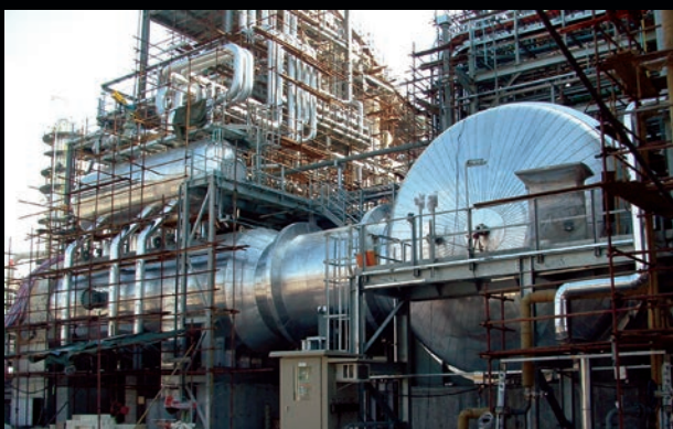
Above: Sulphuric acid cracking unit completely lined by STEULER-KCH refractory materials.
