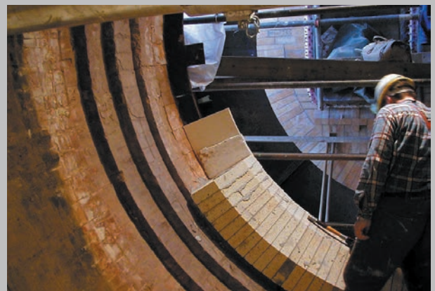
Above: STEULER-KCH also offers erection services thereby ensuring the qualified implementation of the refractory system design
