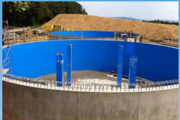
Above: Once the concrete has been poured and cured, all that remains is to seal the joints between the sheets by welding
