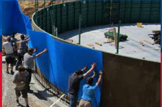
Above: Prior to pouring the concrete, the polyethylene bands are laid in the wall formwork and joined with sections
