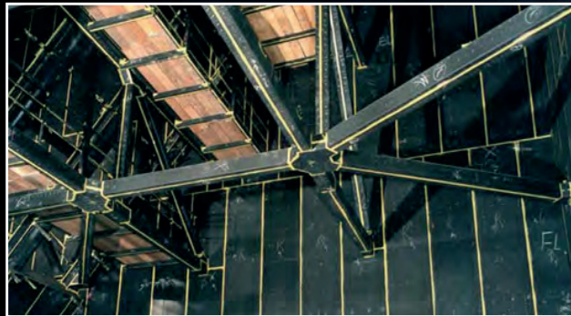
Rubber lining in a flue gas scrubber.
