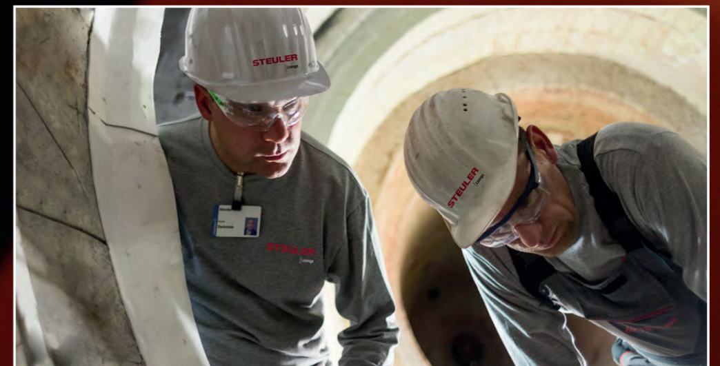
Whether providing supervision or installation with in-house technicians – Steuler's specialists are your guarantee for reliable installation.
