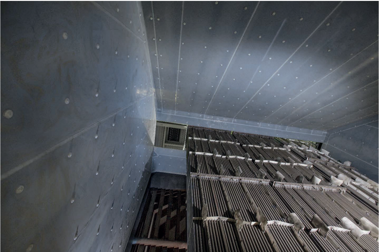
Lining of the flue gas duct (nearly 6 m in diameter) in the Mannheim power station with BEKAFLON from STEULER-KCH. The heat exchangers can be seen in the bottom-right of the picture.
